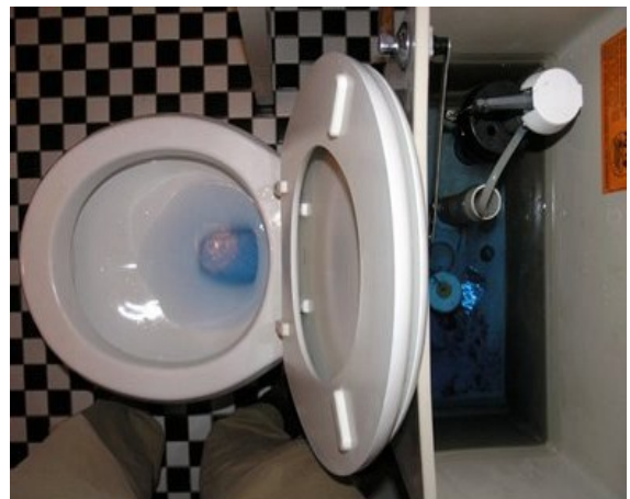
Toilet going through the food coloring test. This one has a leak!
